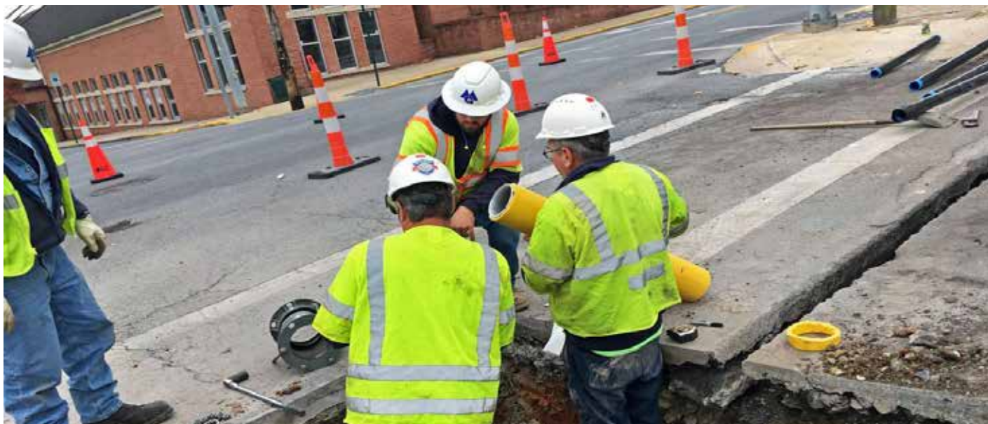
A gas company crew works to repair a gas line damaged by a contractor working on W. Stephan St. in Martinsburg, West Virginia.
