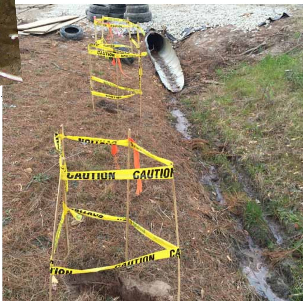
Three pot holes have been made along the path of this buried utility, meaning it could be intersecting another line somewhere down the path.
